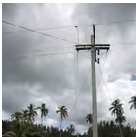
Figure 3: Village connection to the electricity grid facilitated by income received from labour contracts
