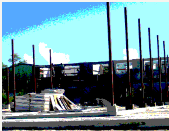
Figure 10. Building the coconut vegetable oil plant for fuel at Kavieng, New Ireland. Emirau (Papua New Guinea)
